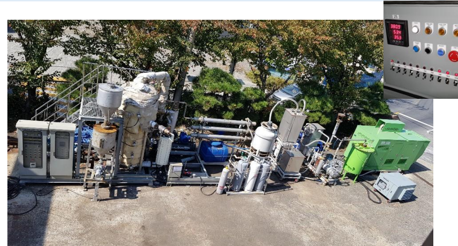
<Two-Stage Biomass Gasification & Gas Engine Power Generation >
